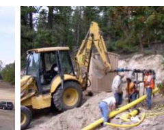
Branson, MO Regulator Station
