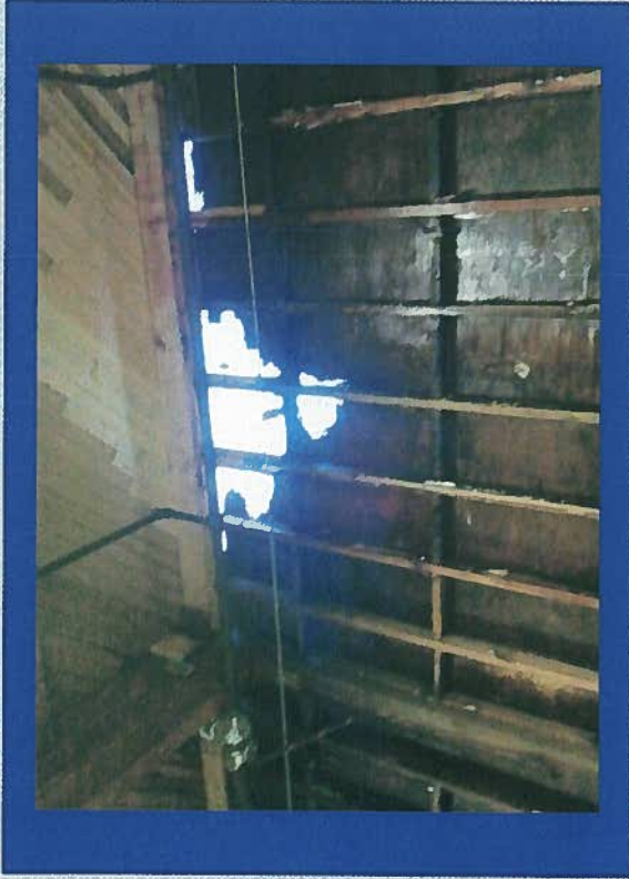
Rotten plywood sheathing on facility walls.
