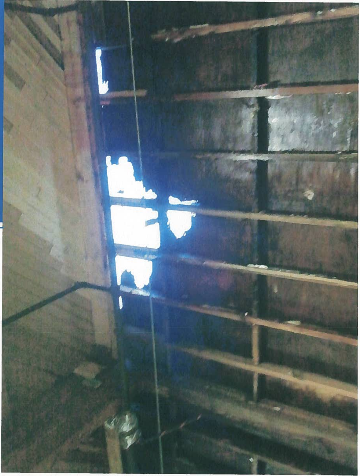
Detail of rotten plywood sheathing: West Wall.
