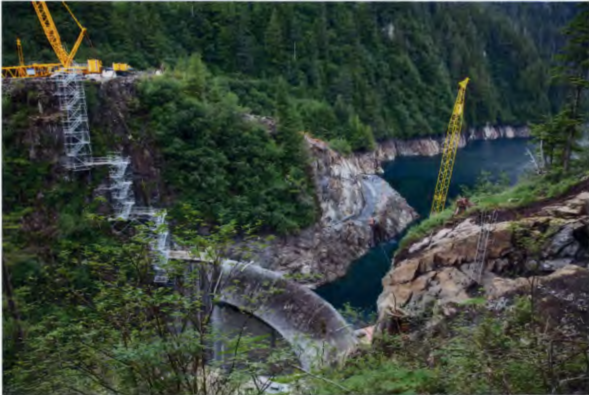
Figure 3. Intake Portal and Right Abutment, Blue Lake Tunnelers have completed 700 of 829 feet of the intake tunnel.
