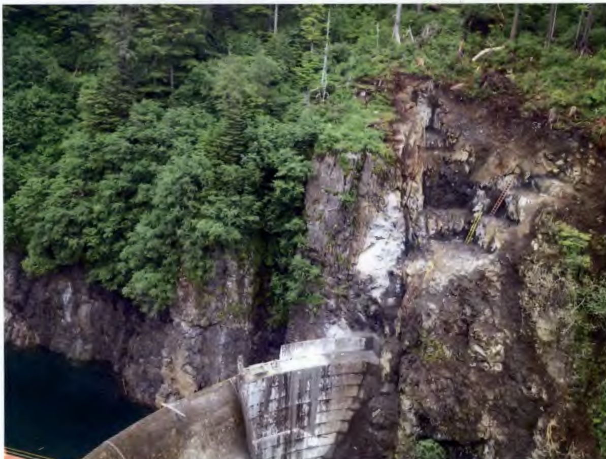
Figure 1. Dam and Left Abutment Area, Blue Lake Tunnelers completed the left abutment thrust block excavation. Work on the keyway began and the first concrete pour was completed on the dam.
