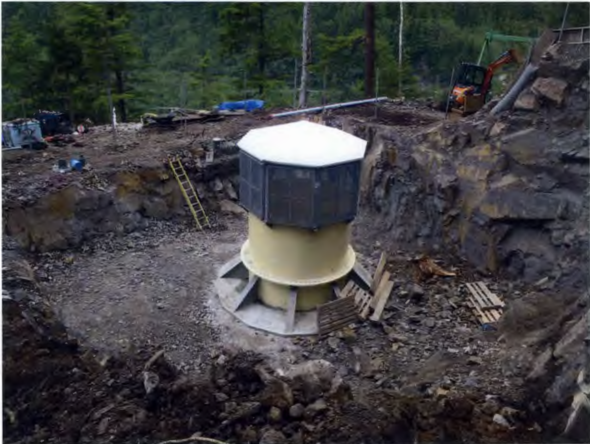
Figure 6. Surge Chamber Top Portal, The small structure over the surge shaft is complete.
