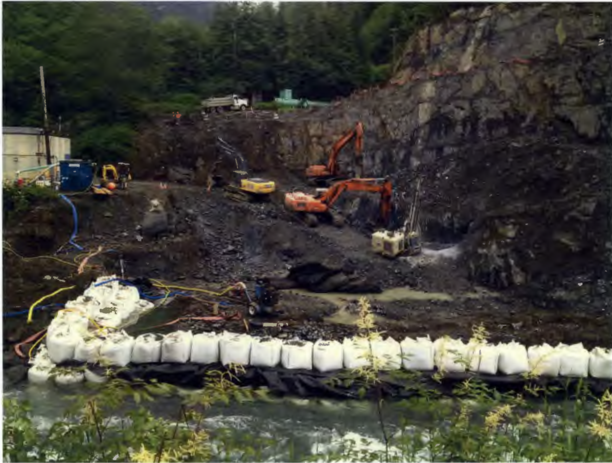
Figure 8. Powerhouse Site, Excavation work in the powerhouse area continued all month with additional work shifts added.
