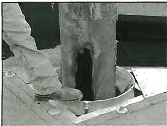
Hole in damaged piling that needs replacing
